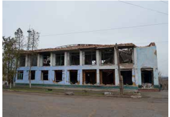
A non-residential building in the center of Snihurivka destroyed by shelling.
