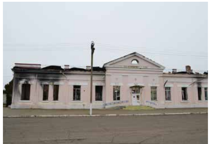
Damaged Snihurivka train station.
